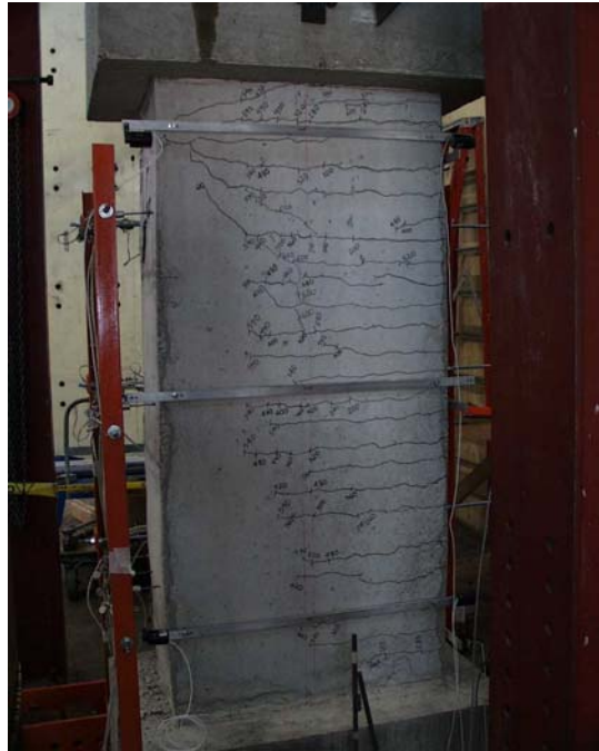
Figure 5.6 Specimen P6: Photo of West Wall at End of Test
