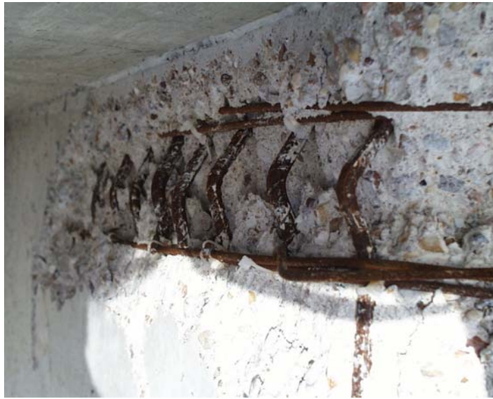
Figure 5.11 Specimen P6: Buckled Longitudinal Reinforcement near the Top of the East Wall
