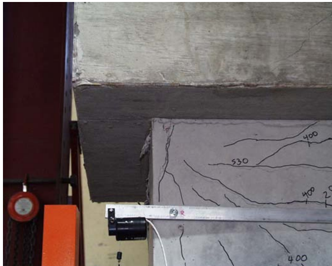
Figure 5.34 Specimen P10: Photo of at Top of Northwest Corner at End of Test
