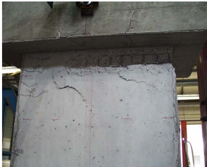
Figure 5.4 Specimen P6: Photo of East Wall at End of Test
