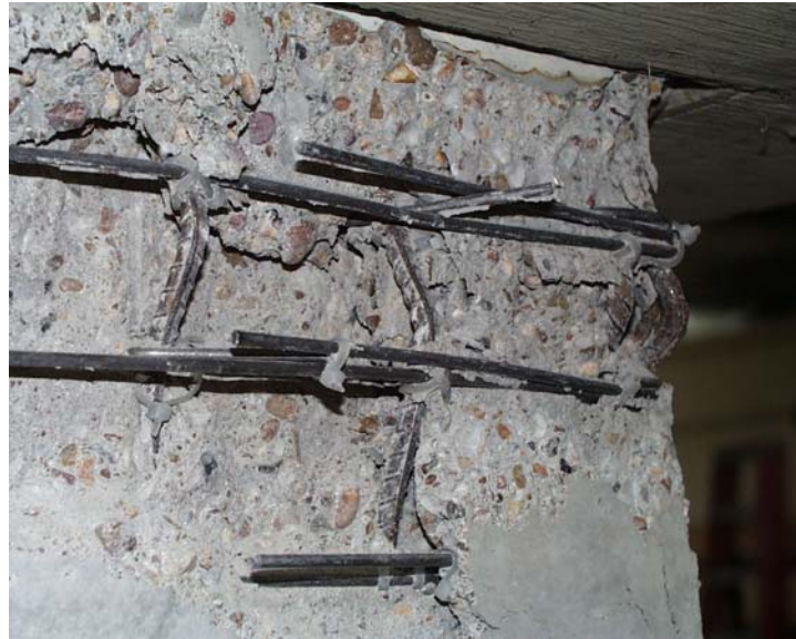
Figure 5.65 Specimen P14: Buckled Longitudinal Reinforcement near Top of East Wall
