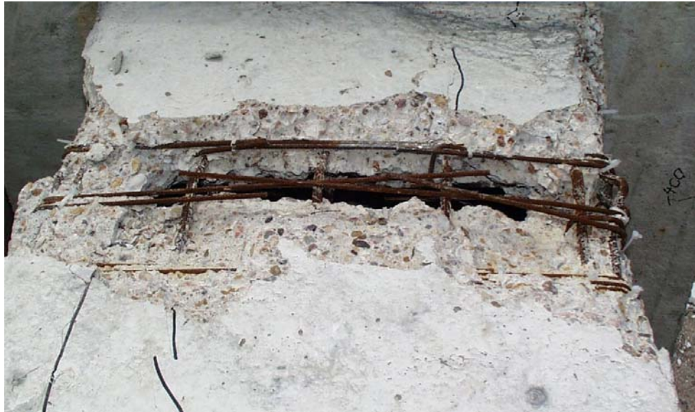
Figure 5.92 Pier P12: Separation of Spliced Transverse Reinforcement along the North Wall
