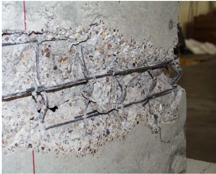
Figure 5.52 Specimen P12: Buckled Longitudinal Bars along the East Wall
