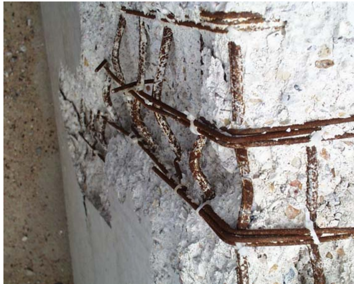
Figure 5.24 Specimen P8: Buckled Longitudinal Bars at the Northeast Corner and in the East Wall
