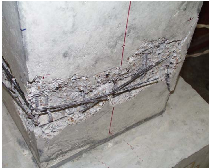
Figure 5.51 Specimen P12: Buckled Longitudinal Reinforcement along the North Wall and Opened Transverse Reinforcement
